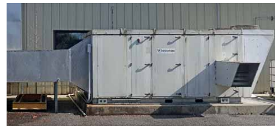
Air conditioning and exhaust air cleaning system with heat recovery (2016)
